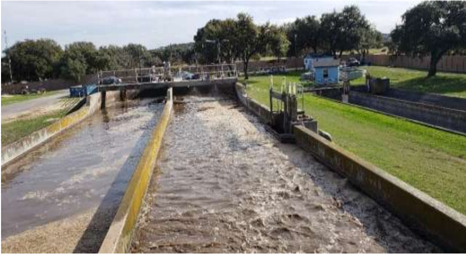
Extended aeration basin at existing WWTP
