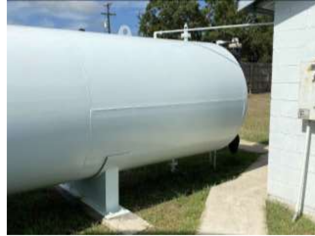
Existing 5,000 gallon hydropneumatic tank at Plant #2
