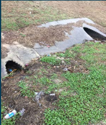
Maintaining and preventing blockage of drainage easements owned by the City
